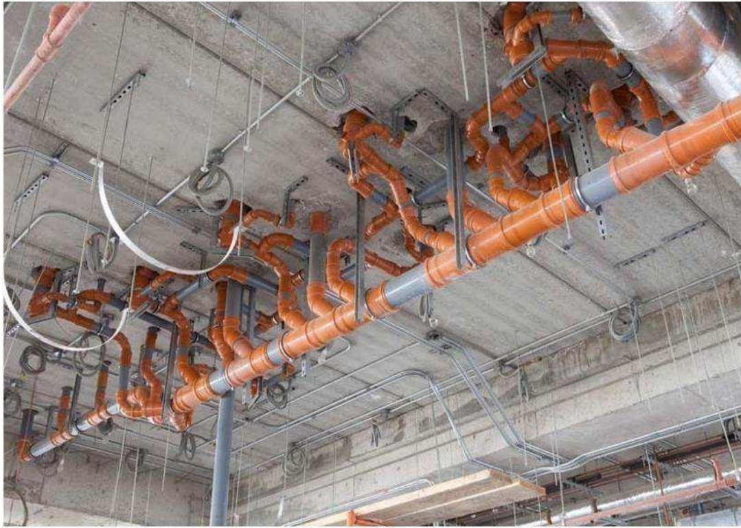
DRAINAGE SYSTEMS MECHANICAL WORKS
